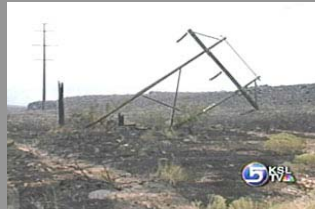
Down Distribution Lines
