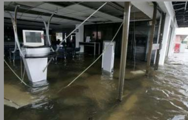
Flooded Credit Union
