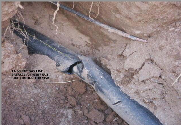
Broken Gas Line
